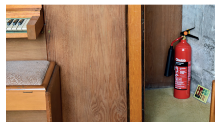
A carbon dioxide extinguisher for electrical fires stationed next to the organ in St Mary’s, Tisbury (Photo: Jonathan Taylor)
