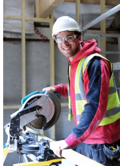
Learning traditional skills through the regeneration of Perran Foundry, Cornwall. Copyright: Toby Weller
