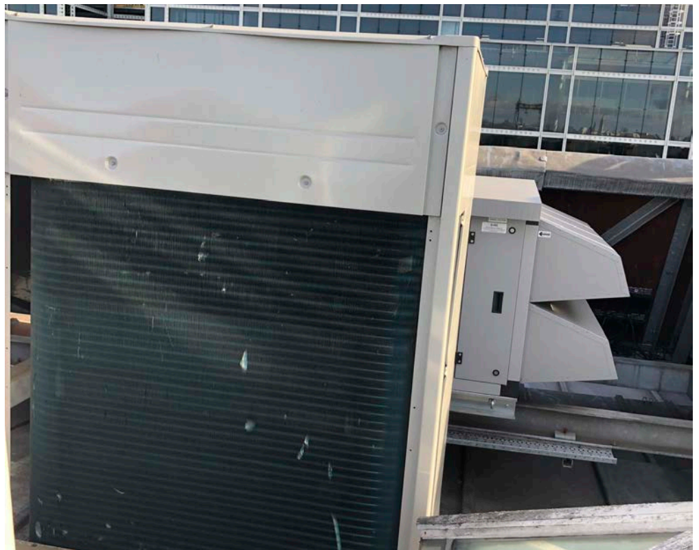
Figure 25: Site 7: ASHP installed on the roof.
