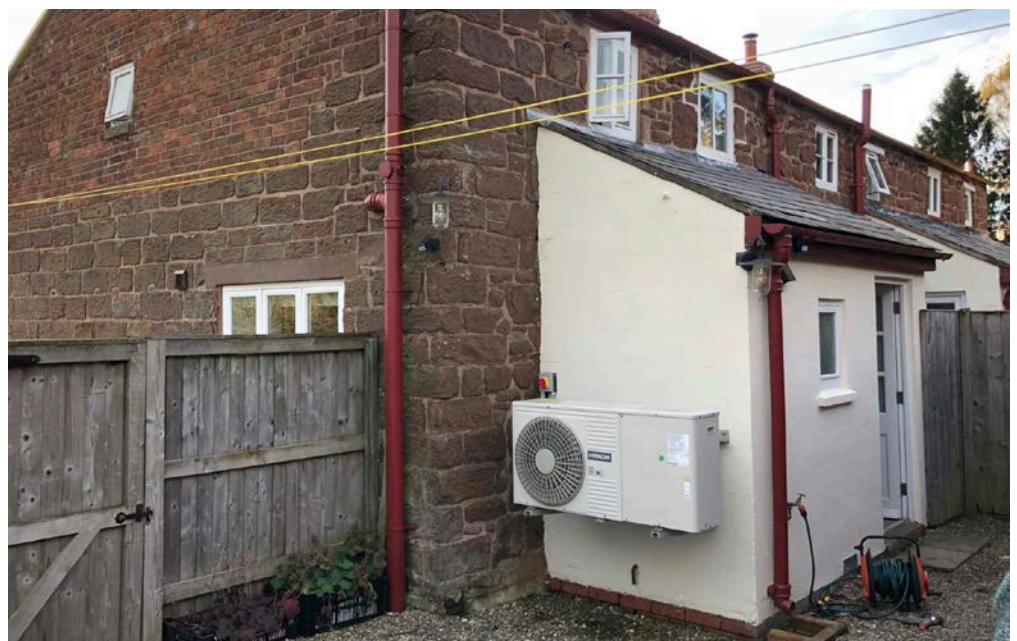
Figure 9: Site 1: ASHP installed at the rear of the house
