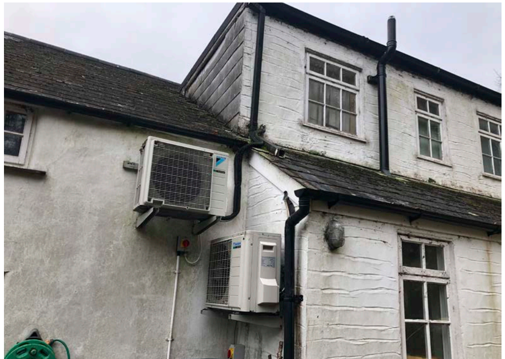
Figure 30: Site 9: The two ASHPs installed at the rear of the building.
