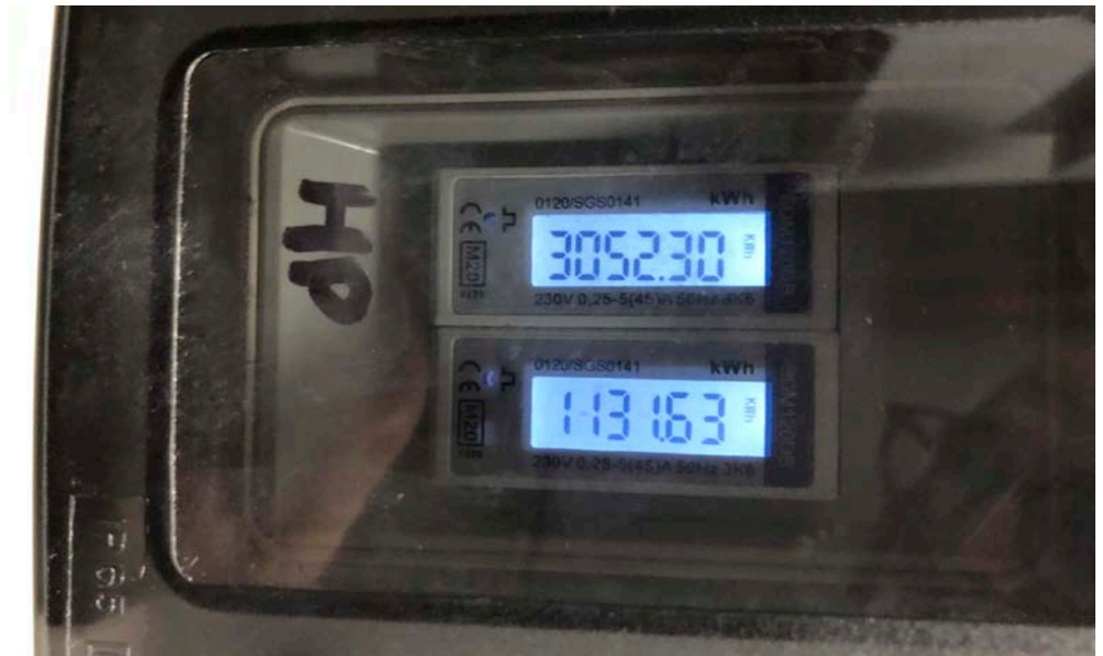
Figure 12: Site 1: Electricity meter showing ASHP kWh in the top display.
