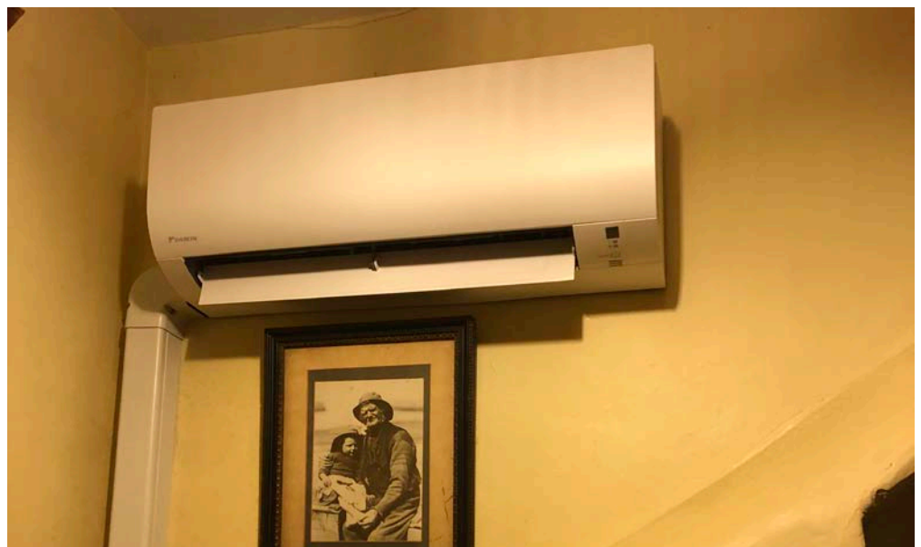
Figure 31: Site 9: A wall-mounted interior condenser unit.
