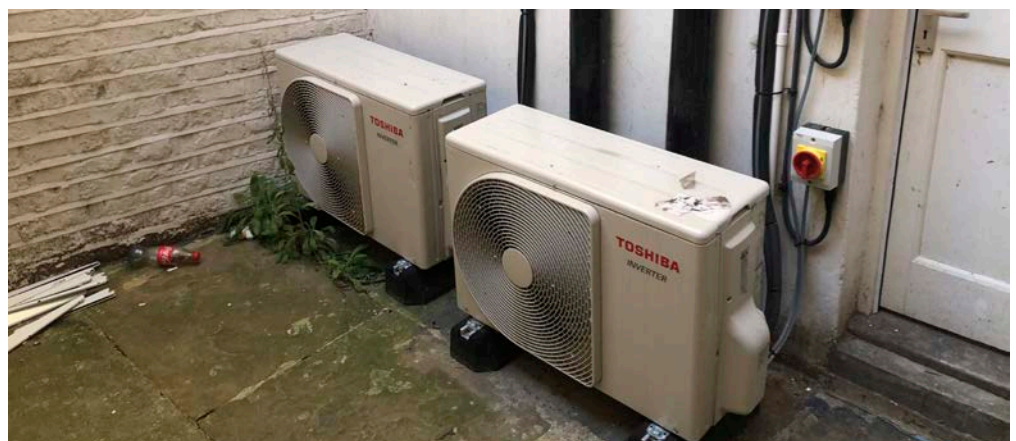
Figure 19: Site 5: The ASHPs in the courtyard.
