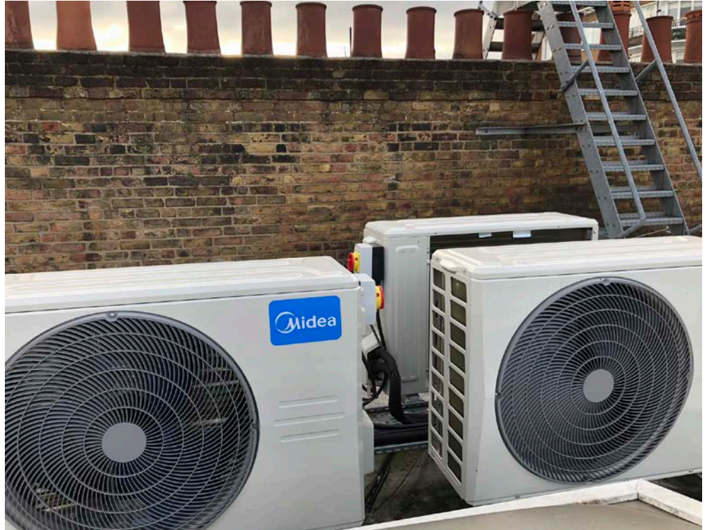
Figure 21: Site 6: ASHPs installed on the flat rooftop.
