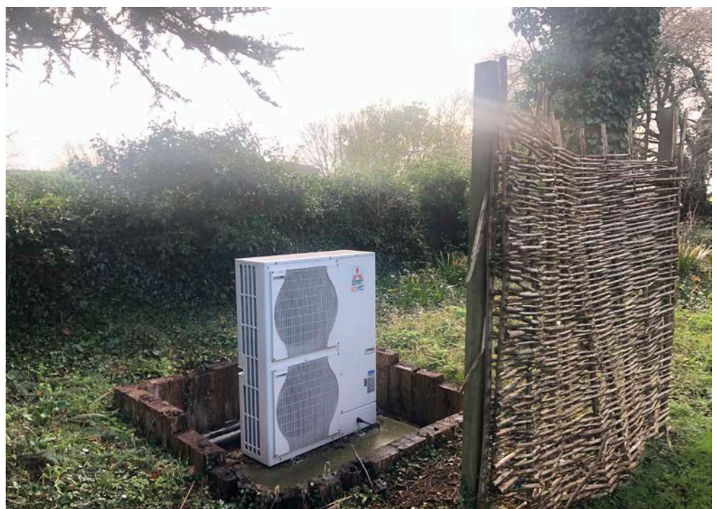
Figure 28: Site 8: The sunken ASHP and the hurdle fence screen.
