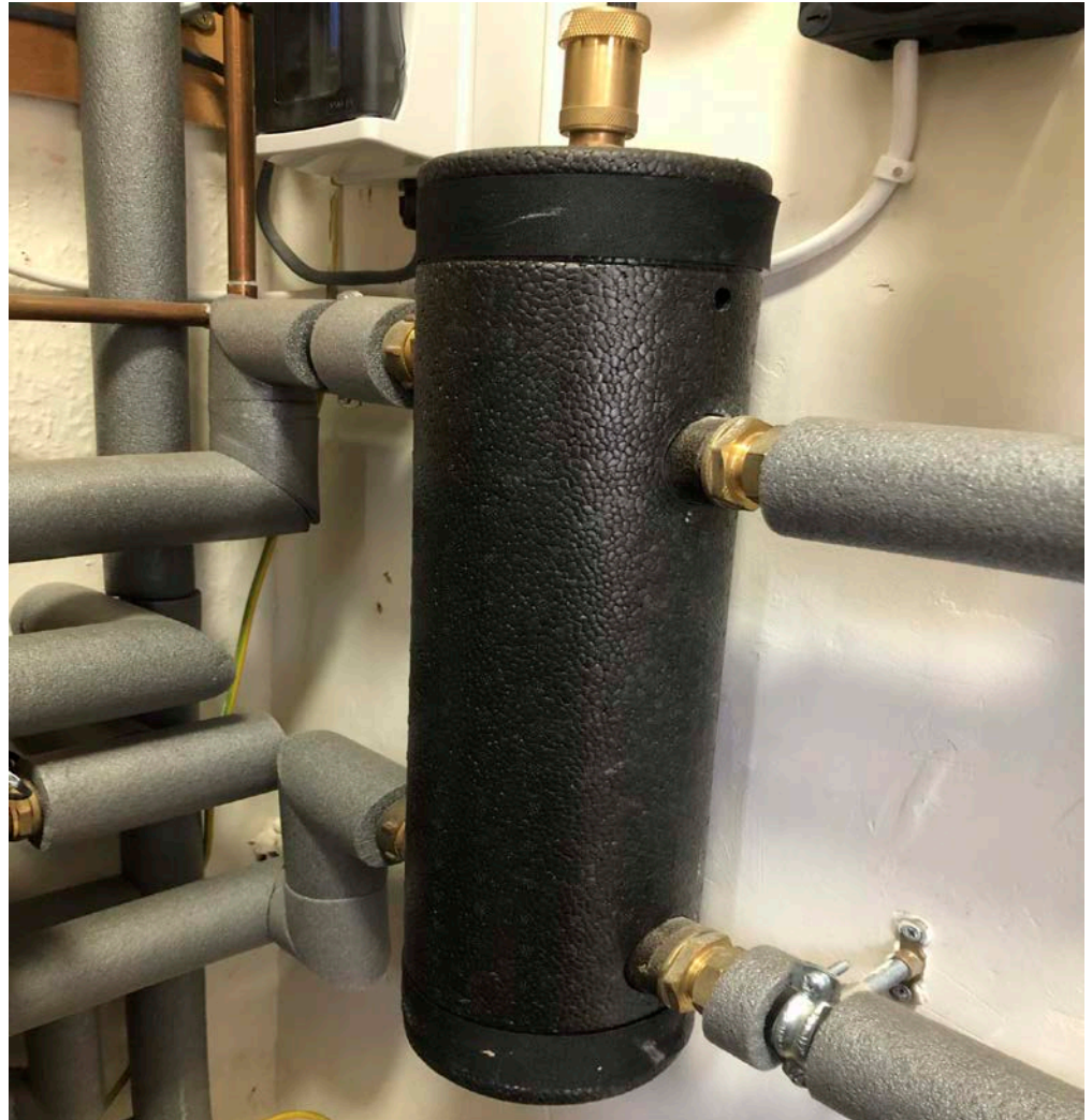
Figure 11: Site 1: The low loss header was not felt to be necessary and was, in fact, detrimental to the efficiency of the ASHP system.
