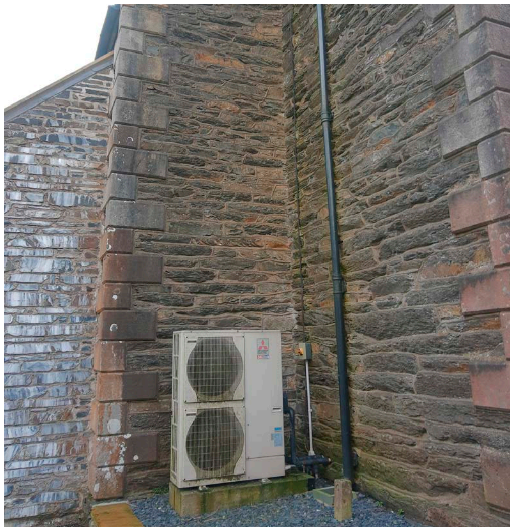
Figure 16: Site 4: The ASHP installed at the rear of the church.
