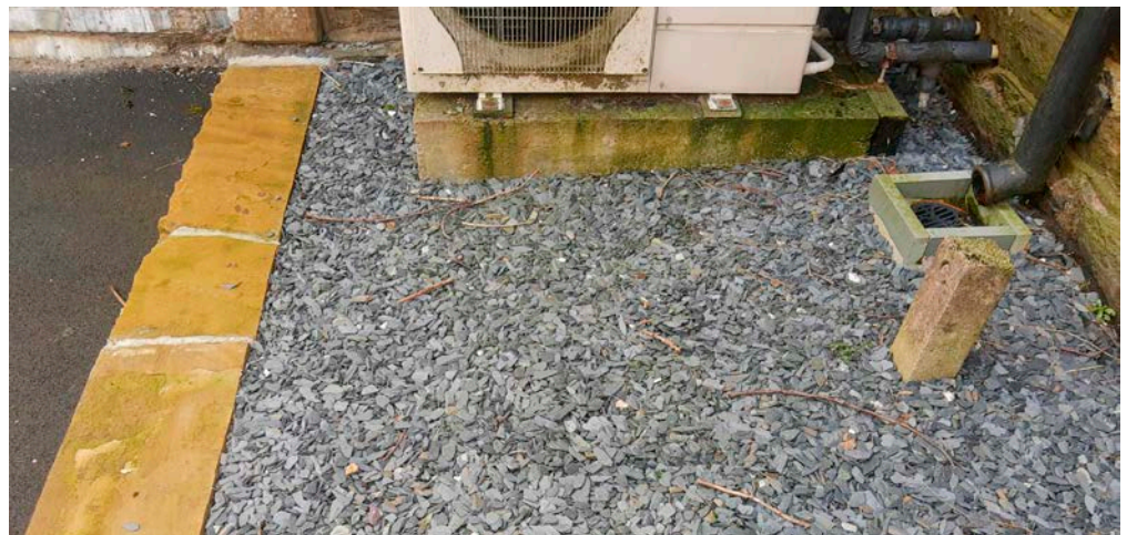
Figure 5: A slate bed at the base of the ASHP allows condensate and defrost water to dissipate safely.
