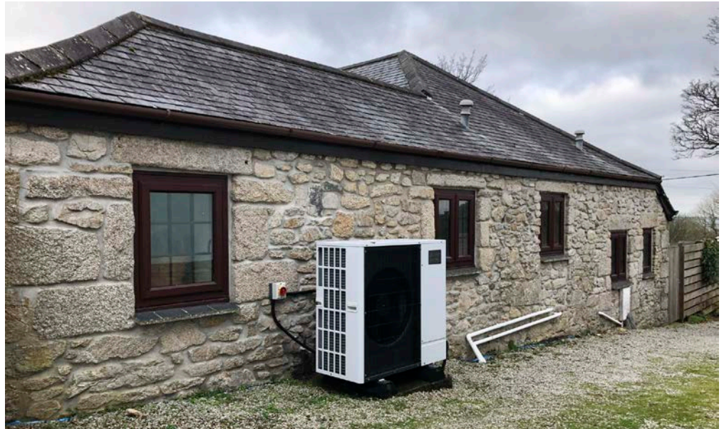
Figure 32: Site 10: The ASHP installed at the side of the converted barn.
