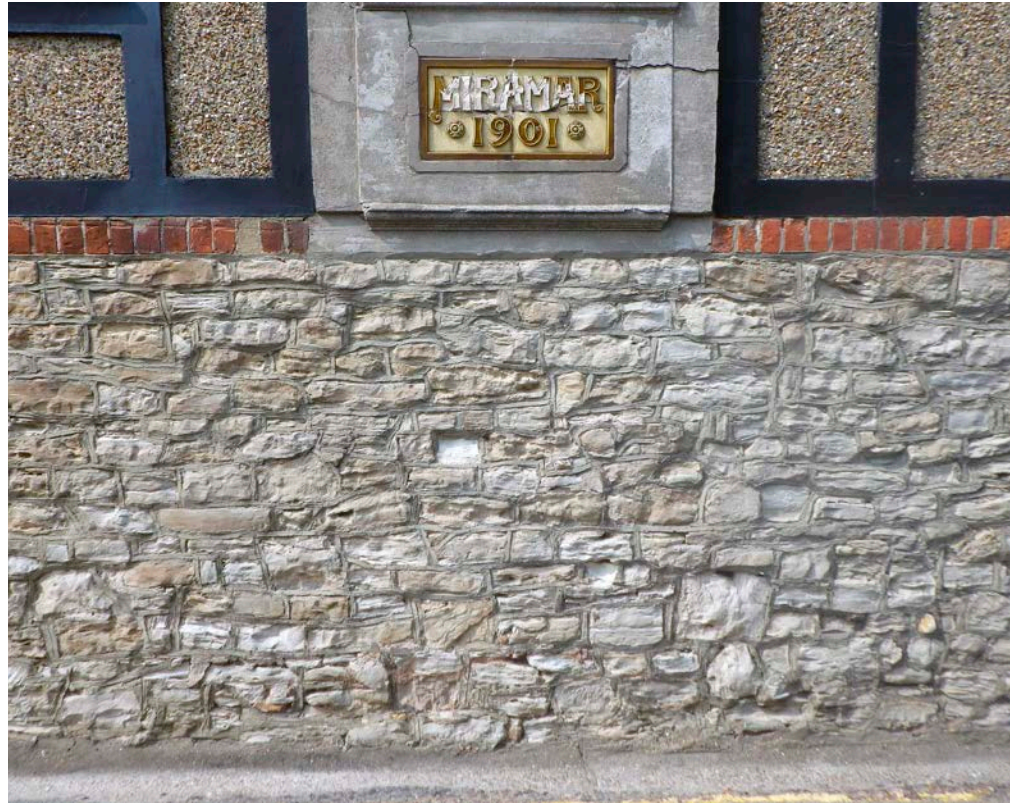
Figure 16: Wall, Seaview Yacht Club, Seaview. Nettlestone Sandstone.
