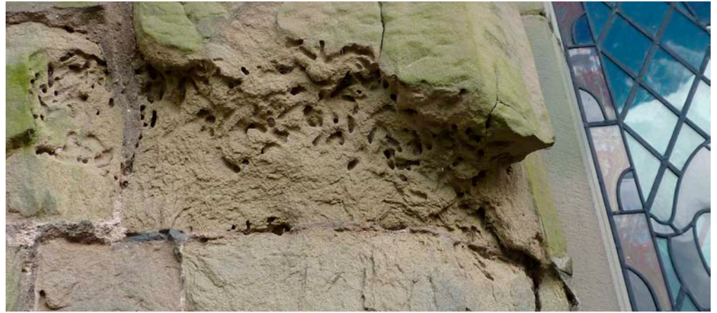
Figure 26: Insect damage to sandstone.
