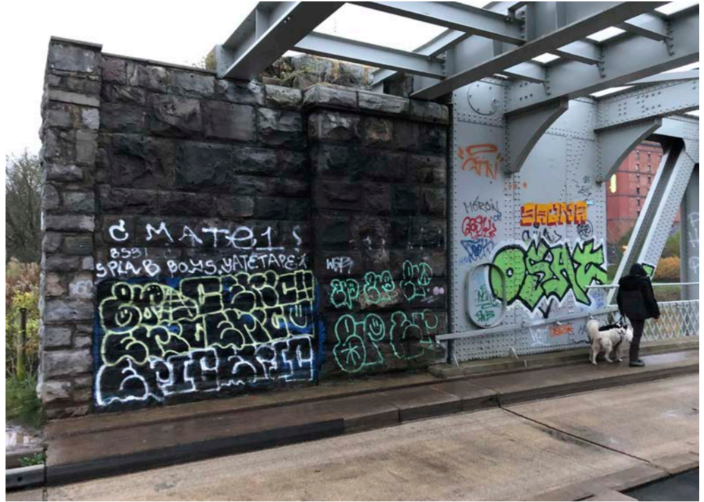
Figure 36: On this bridge, graffiti covers the sandstone masonry piers and the painted iron structure. It is likely that different cleaning methods would be required on each substrate.
