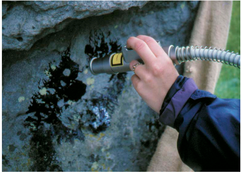
Figure 46: Paint is removed using a Nd:YAG laser. By varying the wavelength of the beam and the area covered by it (by changing the distance of the beam emission to the substrate surface), the optimum fluence (joules of energy per square centimetre) can be achieved.
