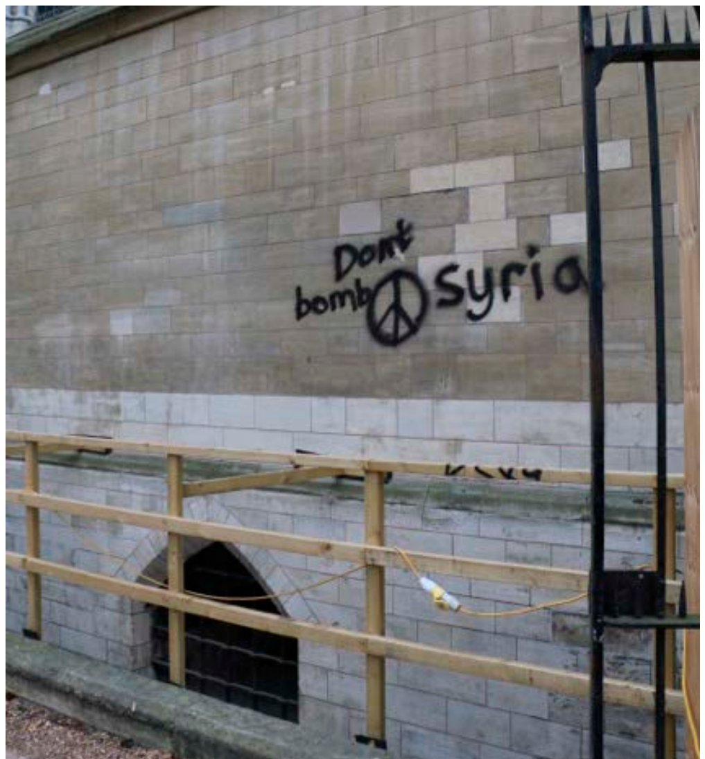
Figure 33: Graffiti was applied to a wall of the Chapter House of Westminster Abbey (a scheduled monument) during an anti-war demonstration in Parliament Square in September 2015. The perpetrator was successfully prosecuted.
