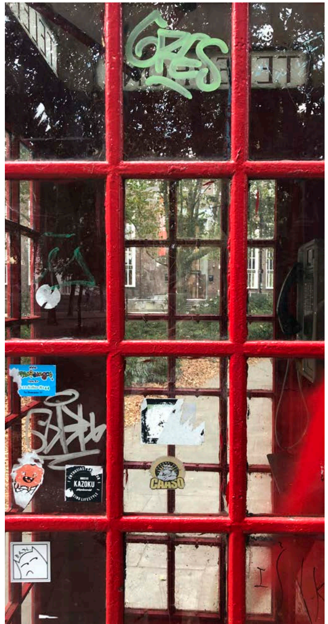
Figure 29 (right): The glass in this red telephone kiosk has been defaced with spray paint, marker pen and adhesive stickers. Glass surfaces resemble ceramic glazes (of faience and tile) in their smoothness and lack of permeability. However, thin glazing is far more vulnerable to damage during graffiti removal, particularly if superheated water is used.
