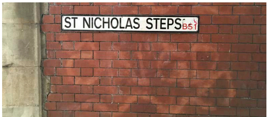
Figure 17: This example of ghosting on brickwork shows where the outline of graffiti remains after removal. This typically occurs when high-pressure mechanical (air abrasive) cleaning follows the outline of the graffiti and results in surface alteration.
