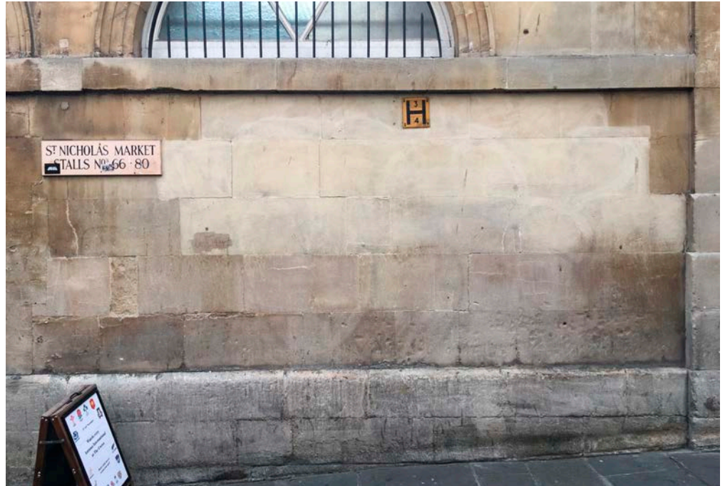
Figure 35: When cleaning stone ashlar, it may be preferable to treat an entire section, respecting architectural lines. The jarring contrasts on this wall could have been prevented by cleaning down to ground level and across to the vertical projections.
