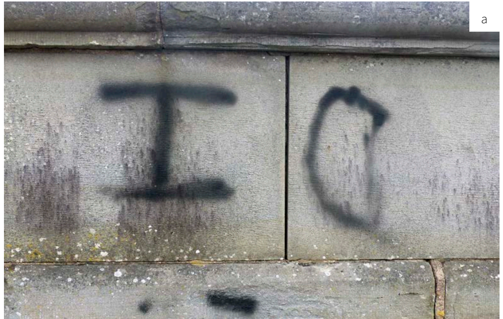
Figure 45: Removal of ghosting is not always fully successful. a) Graffiti on this sandstone was treated with a superheated water spray, graffiti remover gel, ghost remover, acetic acid and hot water rinse. b) Some ghosting persisted.
