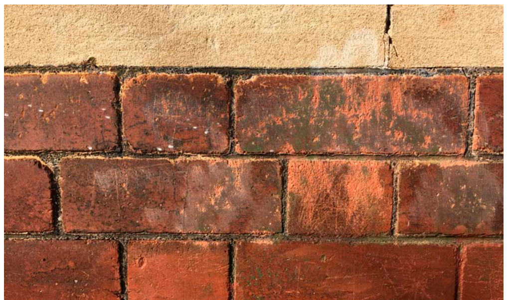
Figure 19: Aggressive mechanical cleaning has damaged these brick faces. Scraping and abrasion have removed the smooth, dark-coloured fireskin, exposing the lighter pinkish and more open-textured body below the surface.
