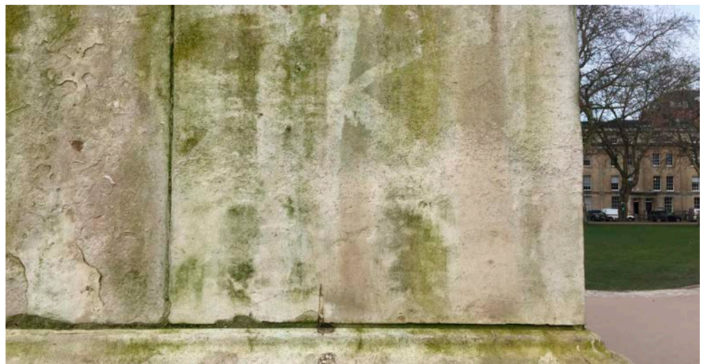
Figure 16: This Portland limestone plinth shows ghosting. The outline of graffiti remains legible several years after the original graffiti was removed, even where re-soiling and green organic growth have occurred on the surface.
