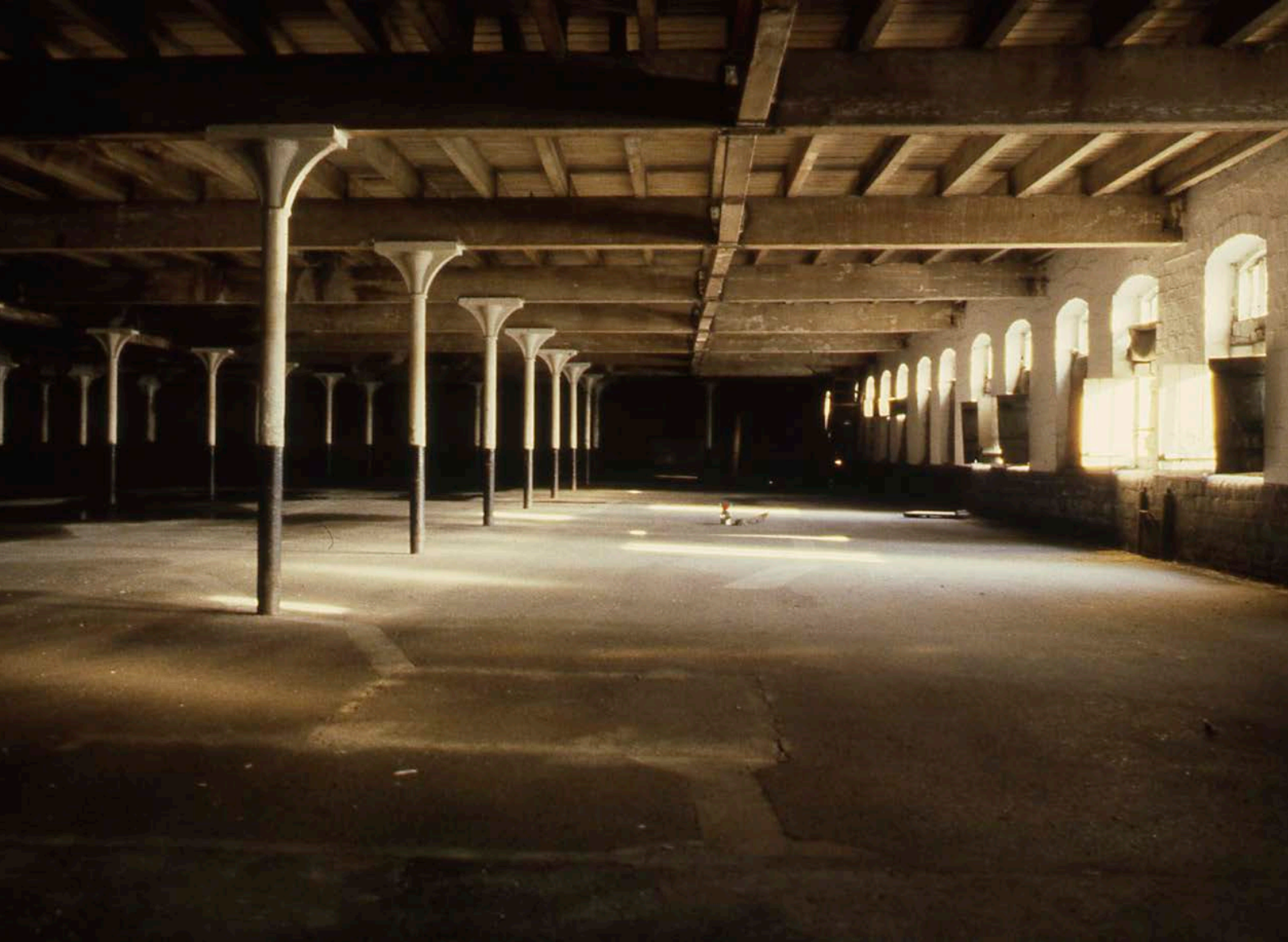
Above: Malthouse, Sherwood Road, Worksop: large open space of the bottom germination floor. © Amber Patrick
