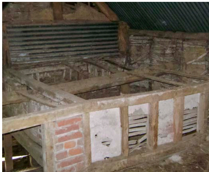
Above: Internal drying floor with low protective walls. Luntley Herefordshire. Hughes. Now demolished.
