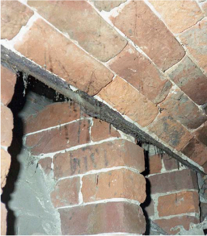
Above: Malthouse, Station Street, Mansfield Woodhouse: the furnace's interior showing the brick spark plate as a vault and its supports which allowing the heat to pass through to the drying floor above. © Amber Patrick
