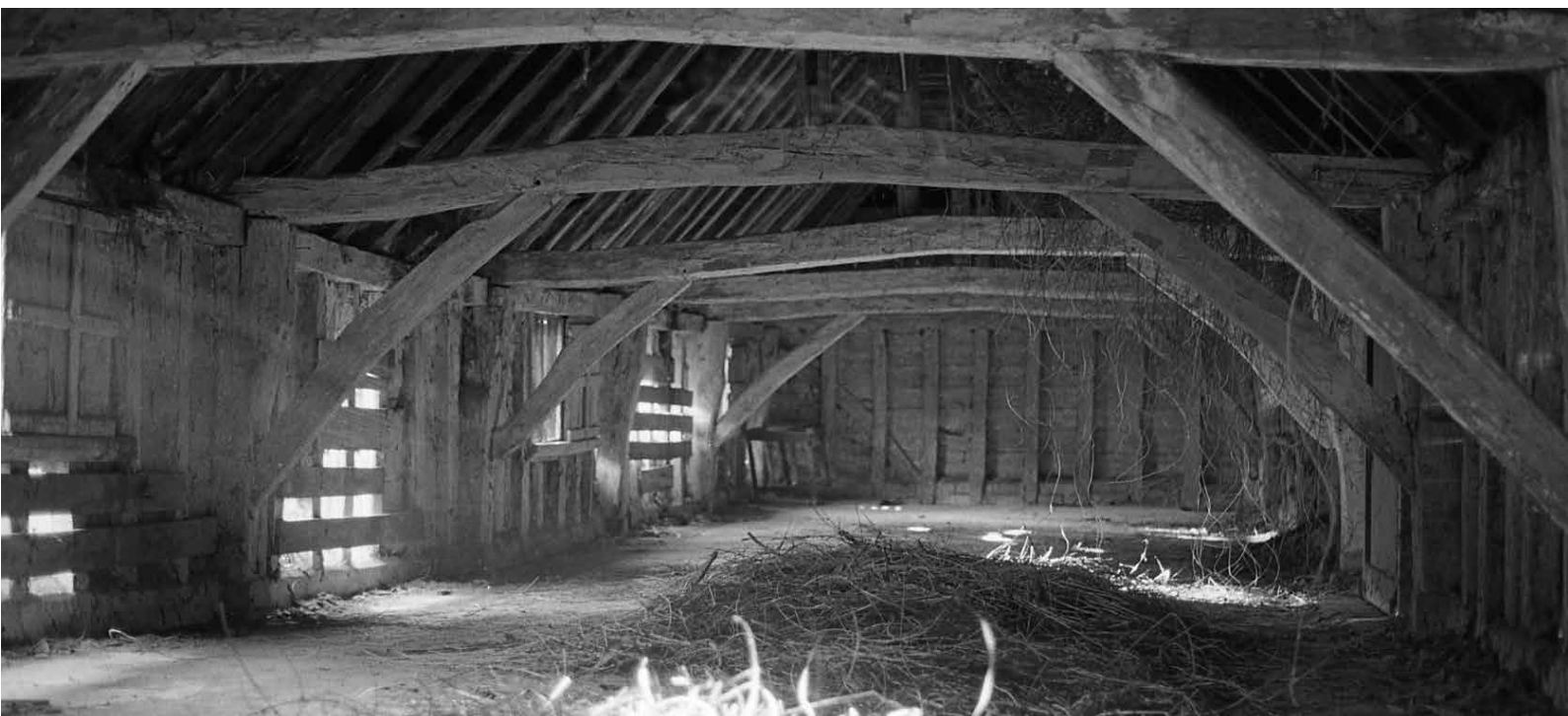
Above: Boyes Croft, Great Dunmow: the first-floor timbers of a 16th century date. © Amber Patrick
