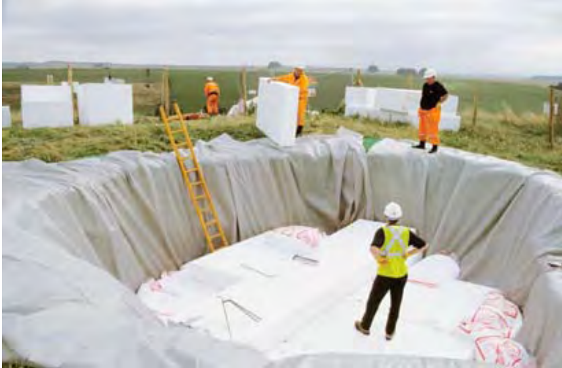
The crown hole was temporarily backfilled with polystyrene blocks in August 2001 before being covered with a layer of chalk
