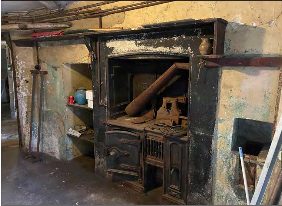
Fig. 73 The range in the north-east basement kitchen [Posy Metz ©Historic England HSLSE09/P8]
