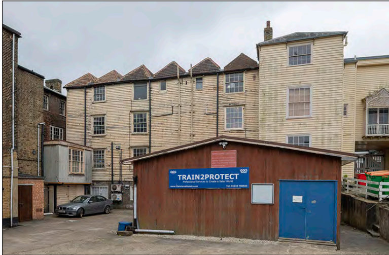
Fig. 48 Rear elevations of Nos 365-371 High Street Rochester [Chris Redgrave ©Historic England Archive, DP289342]
