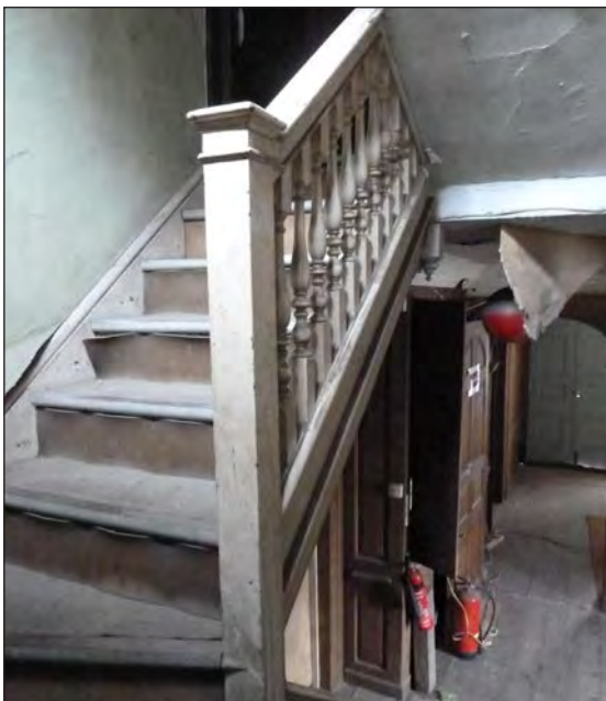
(Above left) Fig 70 The main staircase, ground floor, view from the north-east [Posy Metz ©Historic England HSLSE09/P5]
