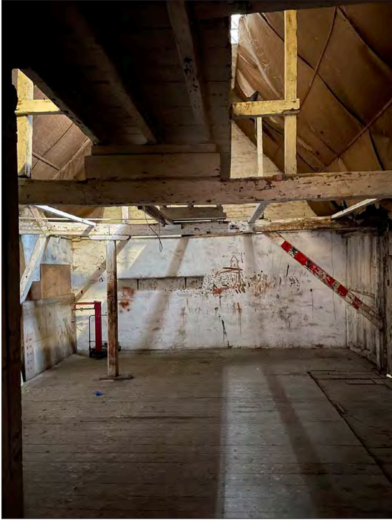
Fig. 76 Interior of the store (formerly the malt store) [Posy Metz ©Historic England, HSLSE09/P9]
